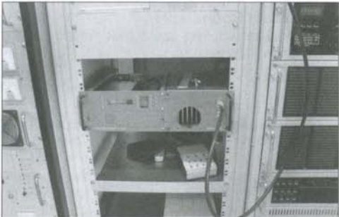
OX3VHF/B beacon rack in GP80KB on 144.4176 MHz
